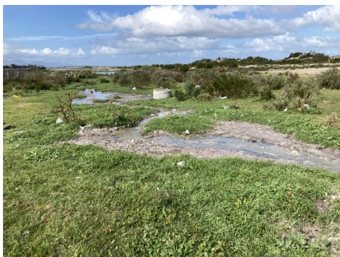
Photo 8.5.5 An overflowing sewer manhole near Mfuleni in the Kuils sub-catchment
