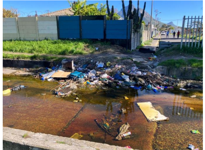
Photo 8.4.2 Accumulation of solid waste in the Bokmakierie Canal just upstream of the Black River confluence, despite City's attempts to reduce access for dumping with fences
