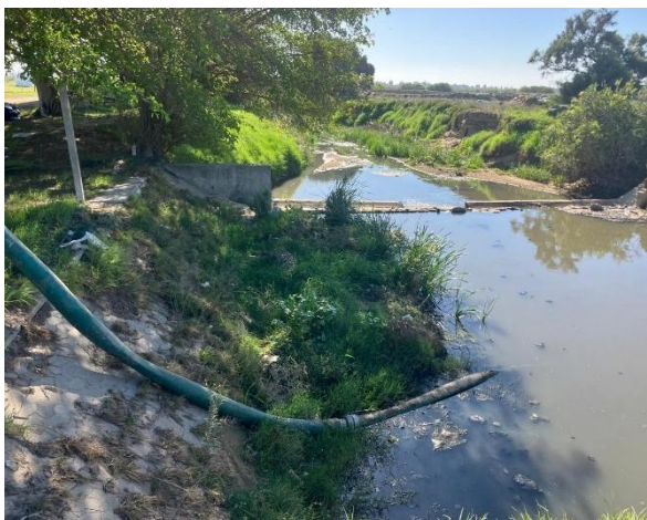
Photo 5.1.3 Sewage overflows into the Theo Marais channel, leading to the Milnerton Lagoon (Diep River Sub-catchment) as a result of prolonged failure of the Koeberg Pump Station
