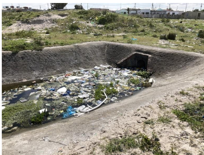
Photo 8.5.6 Accumulation of litter in a major stormwater drain within the Kuils sub-catchment
