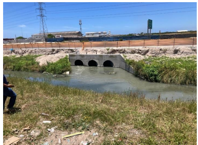
Photo 5.1.4 Outflows of raw sewage enter the Big Lotus River, Zeekoe Catchment, from the Sweet Home and other informal settlements
