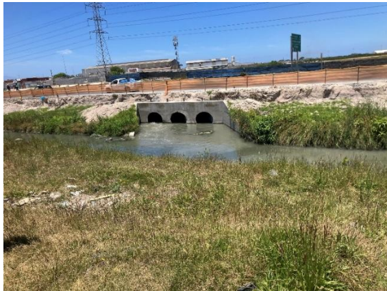
Photo 8.8.3 Significant inflows of polluted water (grey water and raw sewage) into the Big Lotus River from the Sweet Home informal settlement, via the stormwater system (December 2024)
