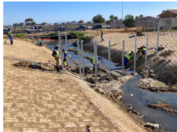
Photo 8.3.6 Waste interceptor devices installed in the Soet Catchment (April 2025) Photo: D. Walker
